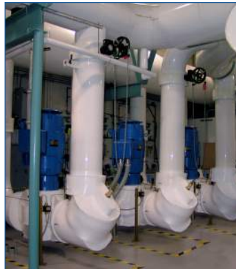
District Cooling Project, Phoenix, U.S.A.
