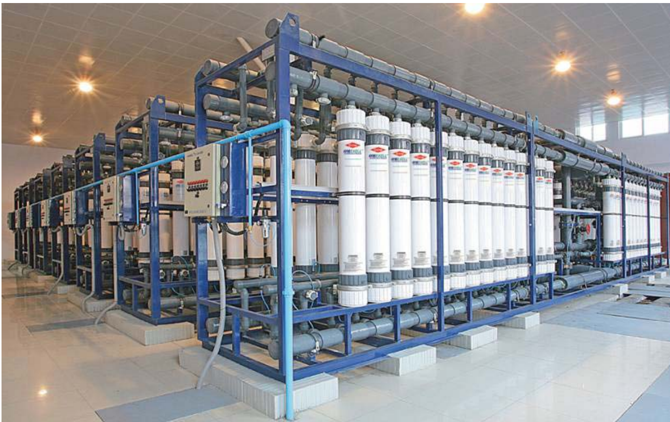
Figure 9: DOW UF Installation using 2860 Modules
