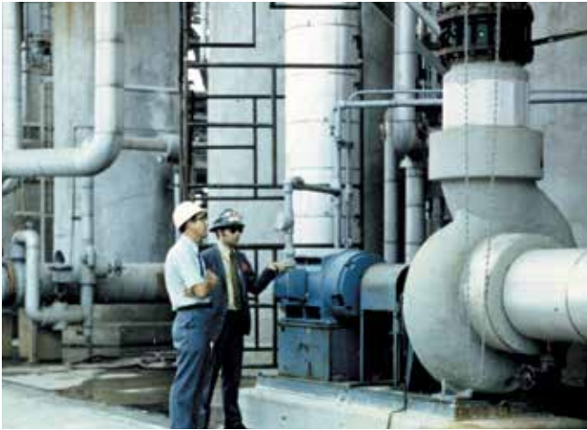
A 3175 installed in a major chemical plant.
