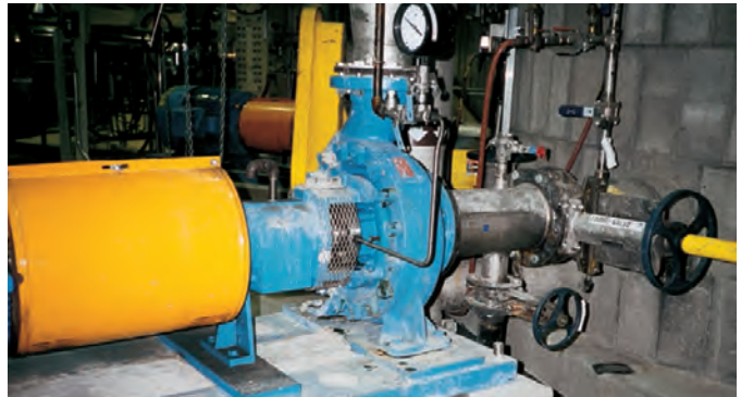
Installation at a North American recycle mill.
