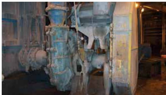
SRL-XT 14×12–36 on Ball Mill Discharge Service
