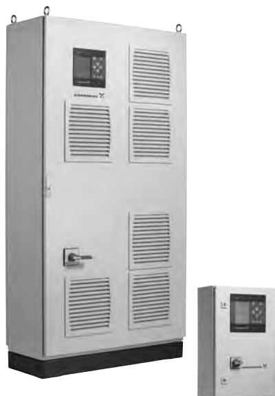
Fig. 6 Floor- and wall-mounted control cabinet
