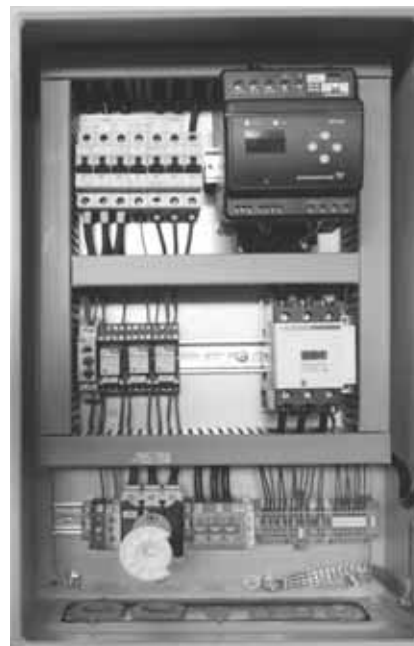
Fig. 13 Inside view of MP 204 panel
