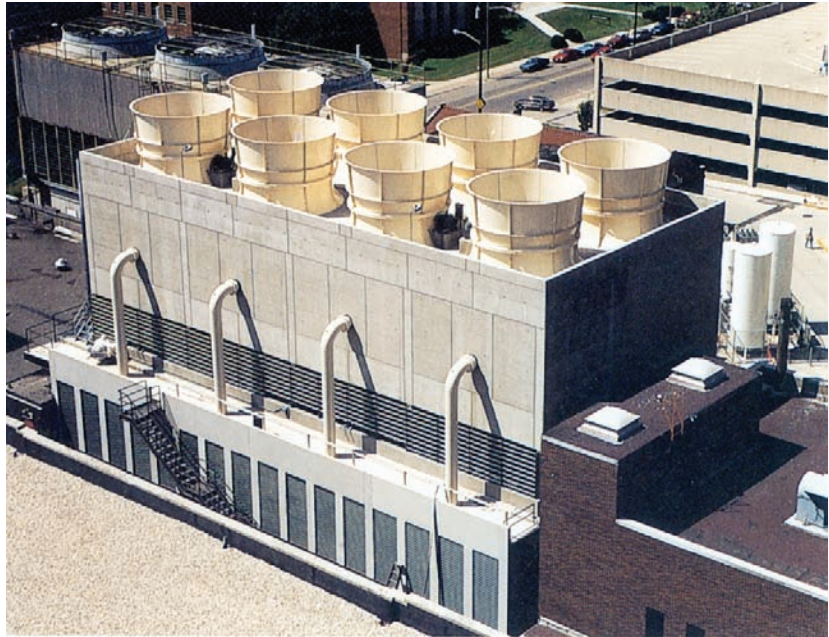
8 Cell Medical Center HVAC system
